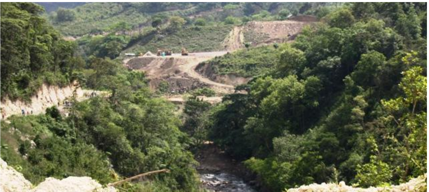
Agua Zarca Dam construction site by the Gualcarque River, Photo by COPINH
